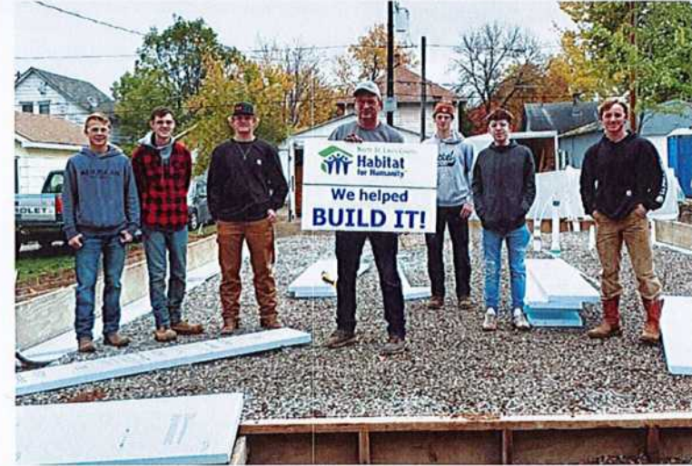
Hibbing High School students, led by Mr. Vessel, preparing the foundation with electrical work being done by Hibbing Community College
