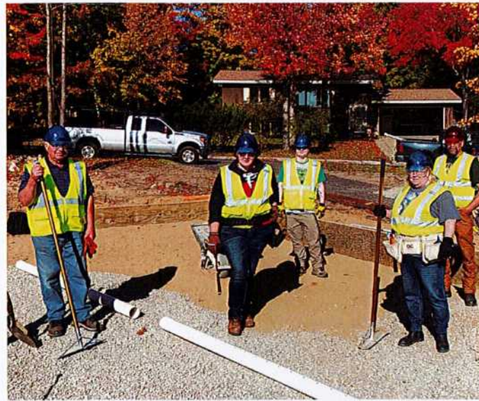
Mesabi Range College Carpentry Class, lead by Leo Lucas, preparing the foundation for the Thrivent Faith Builds home in Gilbert
